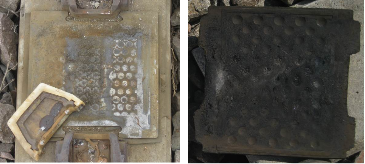
Figure 2.4 Rail pads showing signs of abrasion effects
